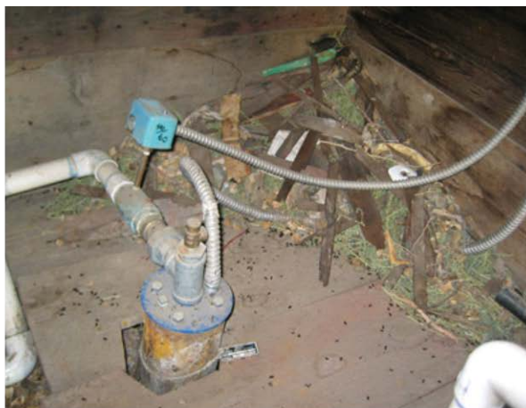
Rat droppings around the wellhead
