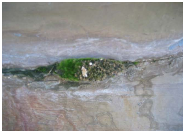
Cracks on a fiberglass tank
