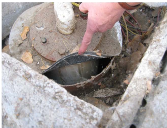
Seal on wellhead not watertight
