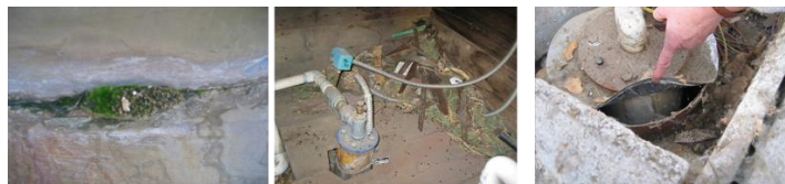
Cracks on a storage tank
